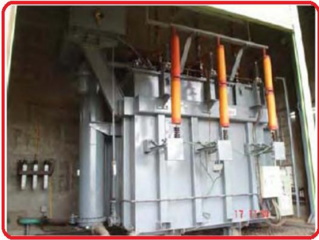
Figure 2.3: Three – phase furnace transformer [11].
