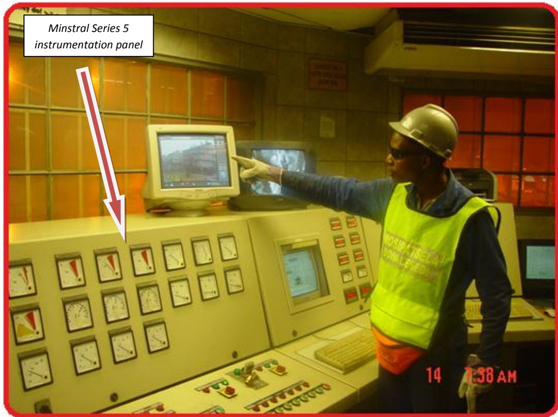
Figure 4.1: Control room panel meters for the measurement of electro-thermal variables (45 MVA SAFs Wonderkop Chrome Processing Plant, SA (2008)).
