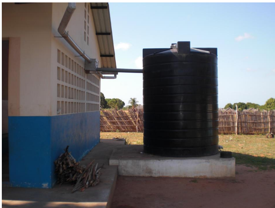
Figure 5.4. Water supply in Mucojo's MWH
