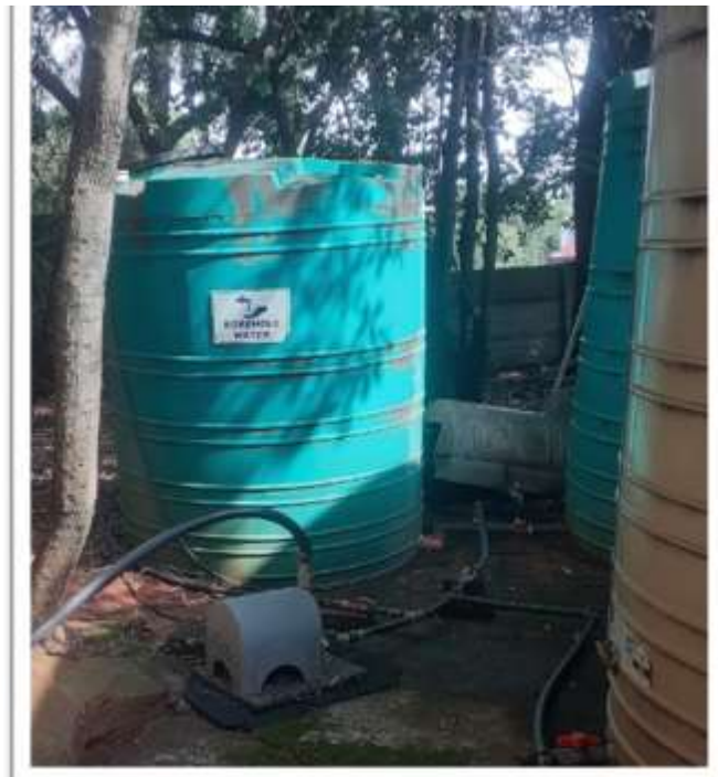
Figure 30: Photograph of Jojo tank connected to borehole system with a water pump. Source: Author
