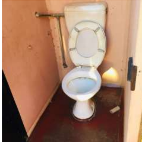
Figure 22: Photograph of a toilet that is connected to the municipality pipelines for household use in Hammanskraal. Source: Author
