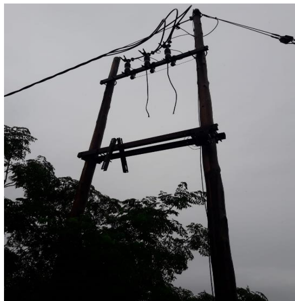
Image 3.1: Pole mounted transformer stolen
