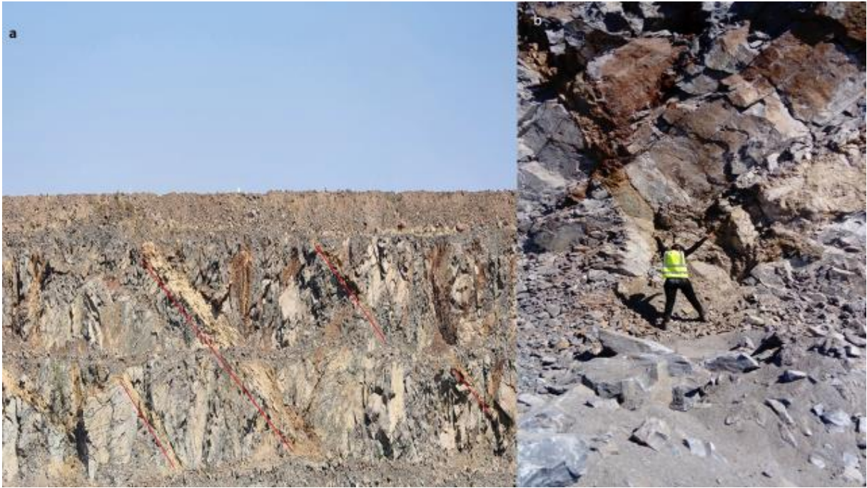
FIGURE 4.1: FAULTING OBSERVED ON THE (A) WESTERN SLOPE FACE AND (B) NORTHERN SLOPE FACE.
