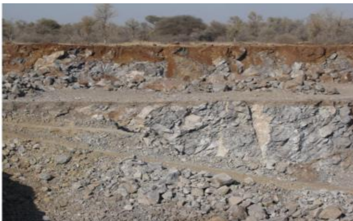
FIGURE 4.8: BURIED SINKHOLE ON THE NORTHERN SIDE OF THE PIT WITH SOIL COVER FILLING UP THE CAVITIES.
