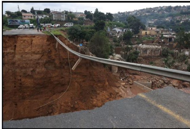
Figure 4.12: A road that has been destroyed in KwaZulu-Natal due to the floods in 2022
