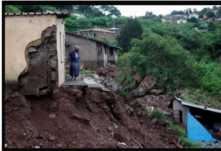
Figure 4.13: A woman standing at her front door of her house after the flood caused flood damage to the surrounding houses
