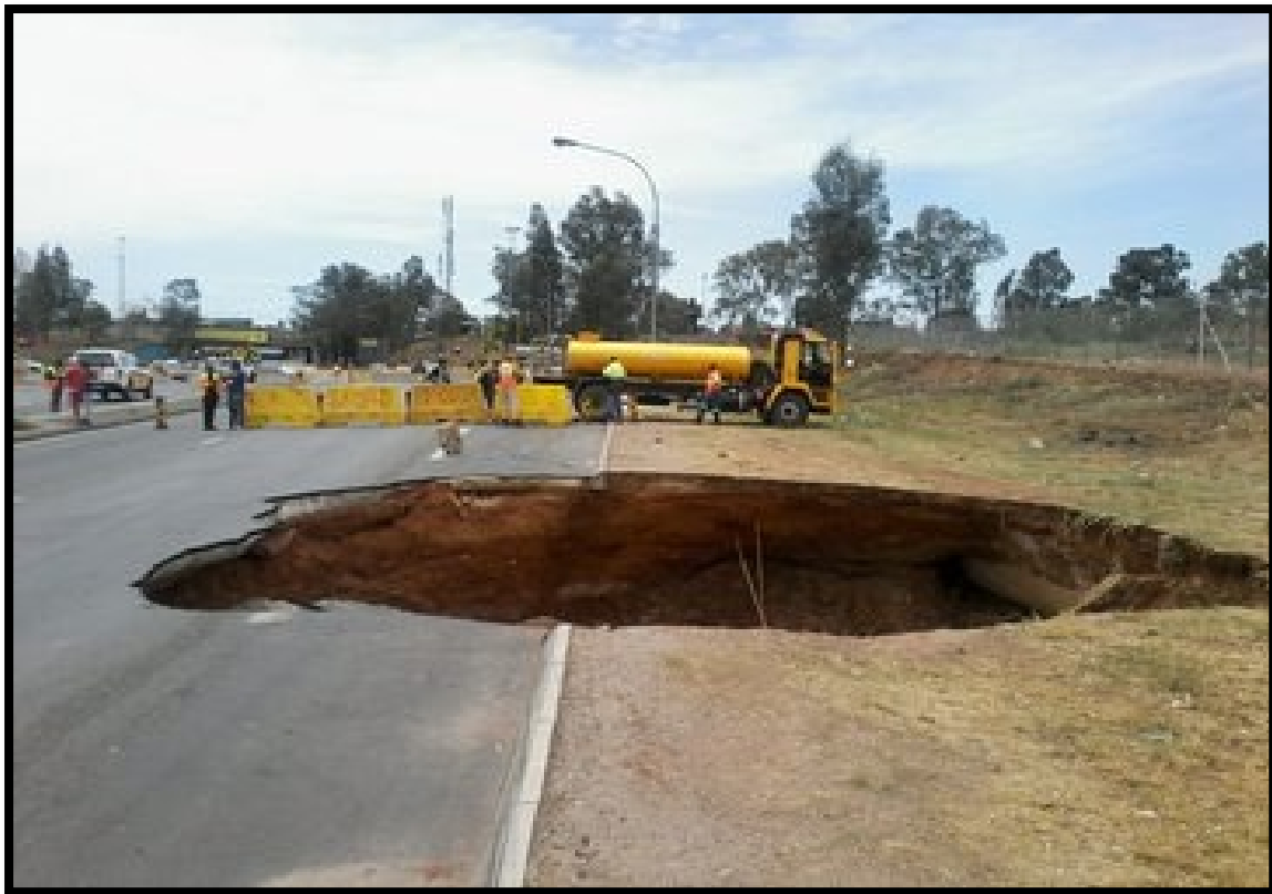
Figure 5.4 Sinkhole in Snake Road, Benoni.
