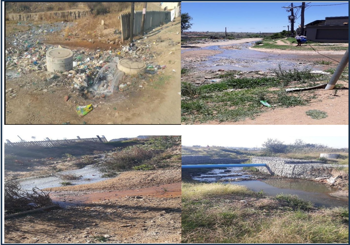
Figure 1.2: Photos taken during site visits showing raw sewage overflowing into Pristine stream (Taken by Mavhungu TC).
