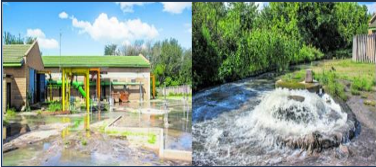
Figure 1.1: Sewage overflowing from Zandspruit pumpstation (Bega,2023).
