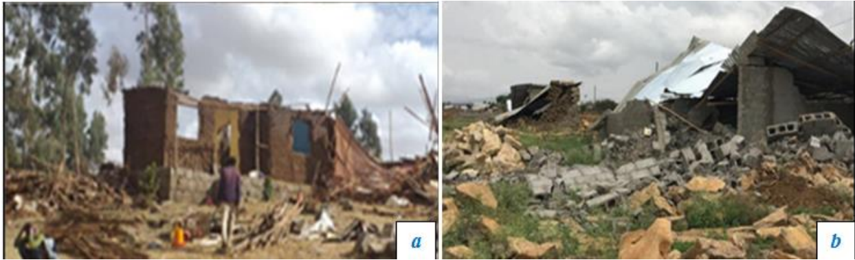
Figure 3.2 (a and b): Continued removal of informal settlement in Ethiopian towns/cities Source: Adopted from ‘Mereja Addis Standard’ and Mereja TV, 2019.
