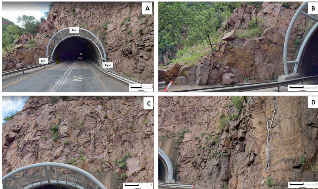
Figure 4.7: GSI rock mass rating on Tunnel Two: (a) tunnel one with all three sides visible, (b) left side of tunnel two, (c) top portion of tunnel two, (d) right side of tunnel two.
