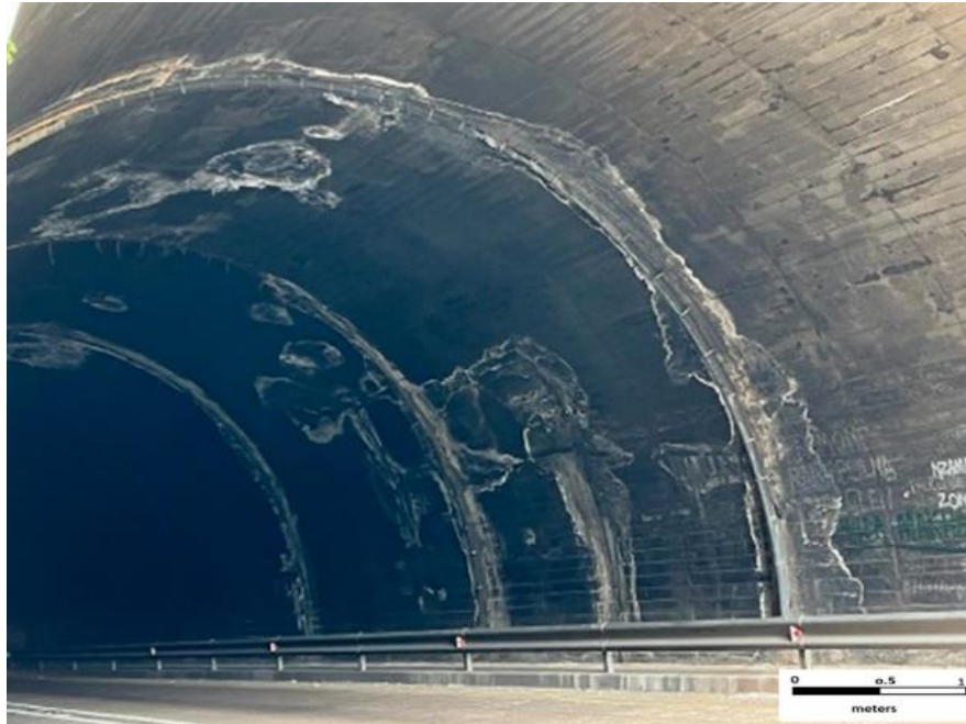
Figure 4.3: Evidence of water seepage in Tunnel One
