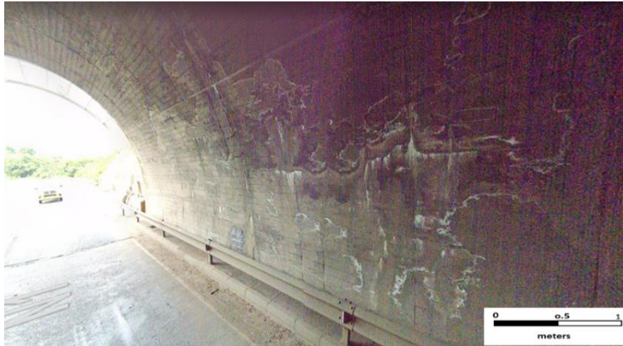
Figure 4.5: Evidence of water seepage in Tunnel Two
