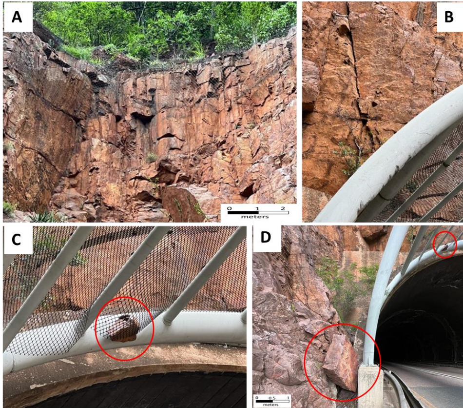
Figure 4.2: Rock mass conditions in the vicinity of Tunnel One: (a) Blocky weathered ground supported with wire mesh; (b) Fractured rock on the top of the tunnel; (c) Evidence of rock fall from the top of the tunnel; and (d) Evidence of rock fall on the left side of the tunnel
