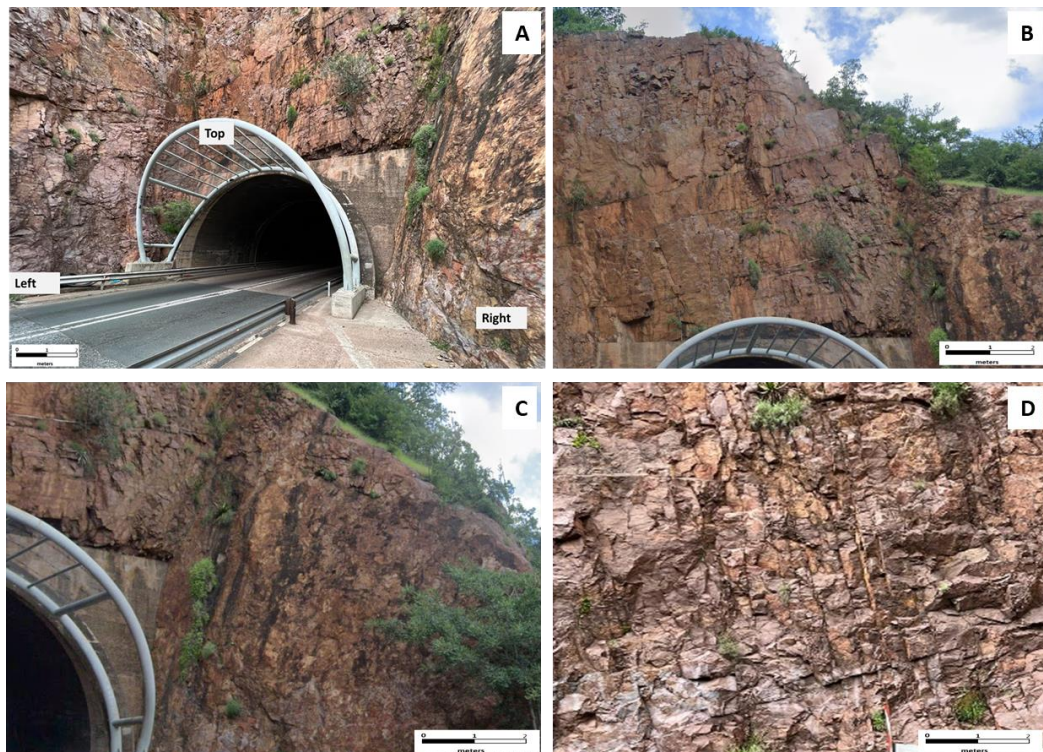
Figure 4.6: GSI rock mass rating on tunnel one: (a) tunnel one with all three sides visible, (b) Top portion of tunnel one, (c) right side of tunnel one, (d) left side of tunnel one.
