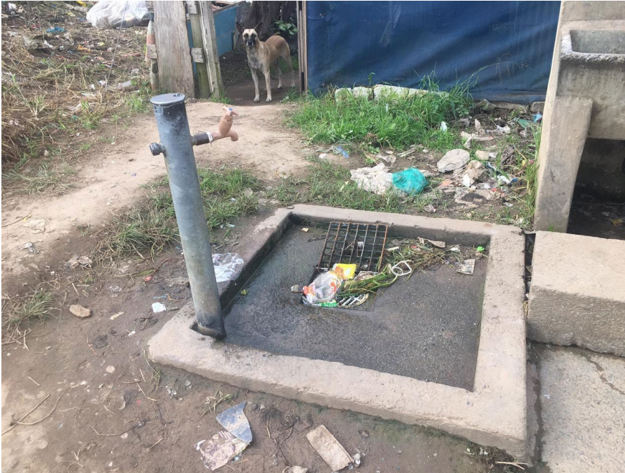
Leaking tap next to the open space
