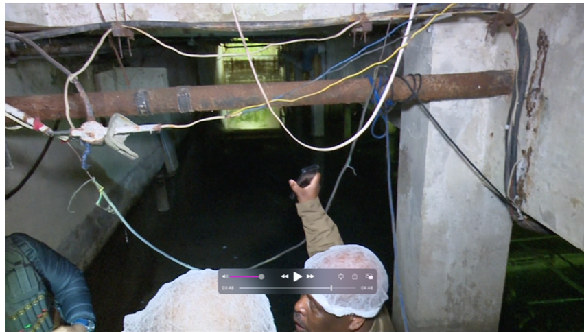
Figure 17: Minister Lamola and officials observing the dilapidated state of some sections of the Johannesburg Correctional Centre (Republic of South Africa. Department of Correctional Services 2019).
