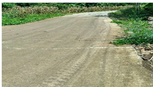
Figure 4. Road condition to Pencong Hot Springs
