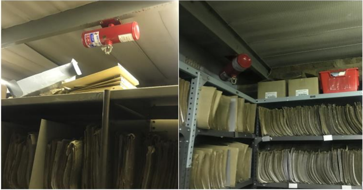
Figure 4-39: Fire extinguishers in archives room (Photographer: Researcher 2020)
