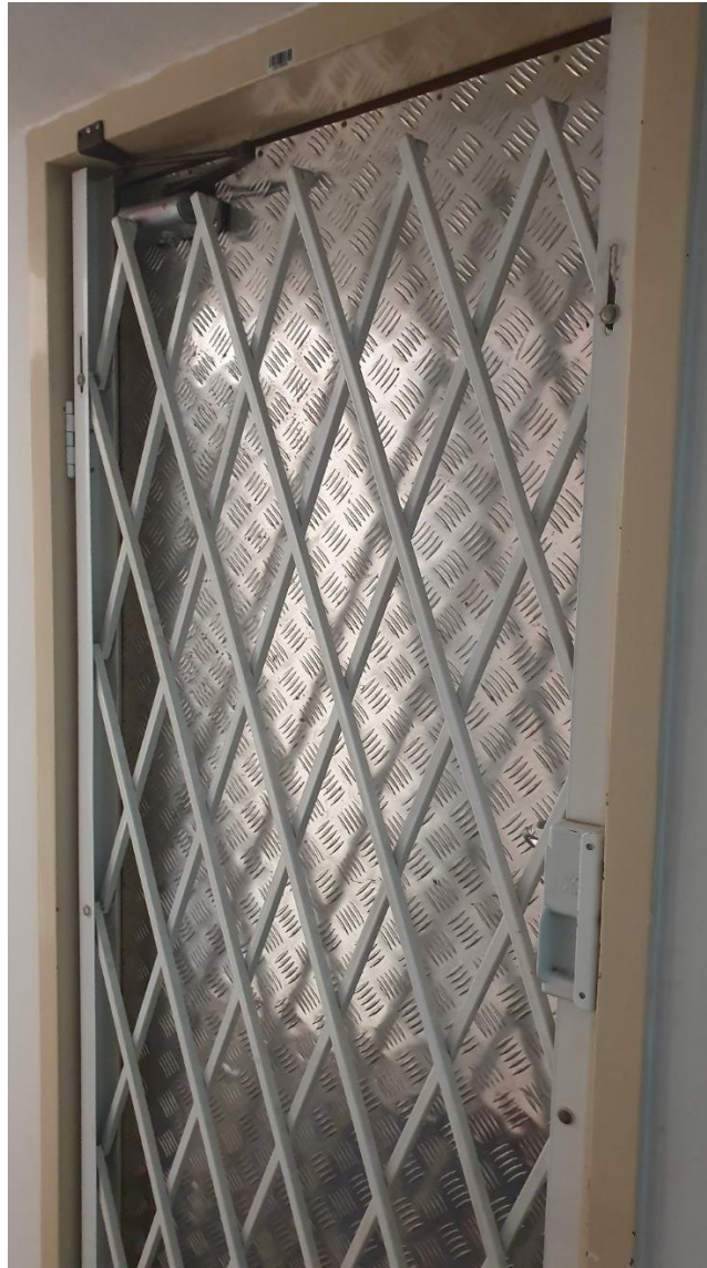
Figure 4-44: New server room door (Photographer: Researcher 2020)
