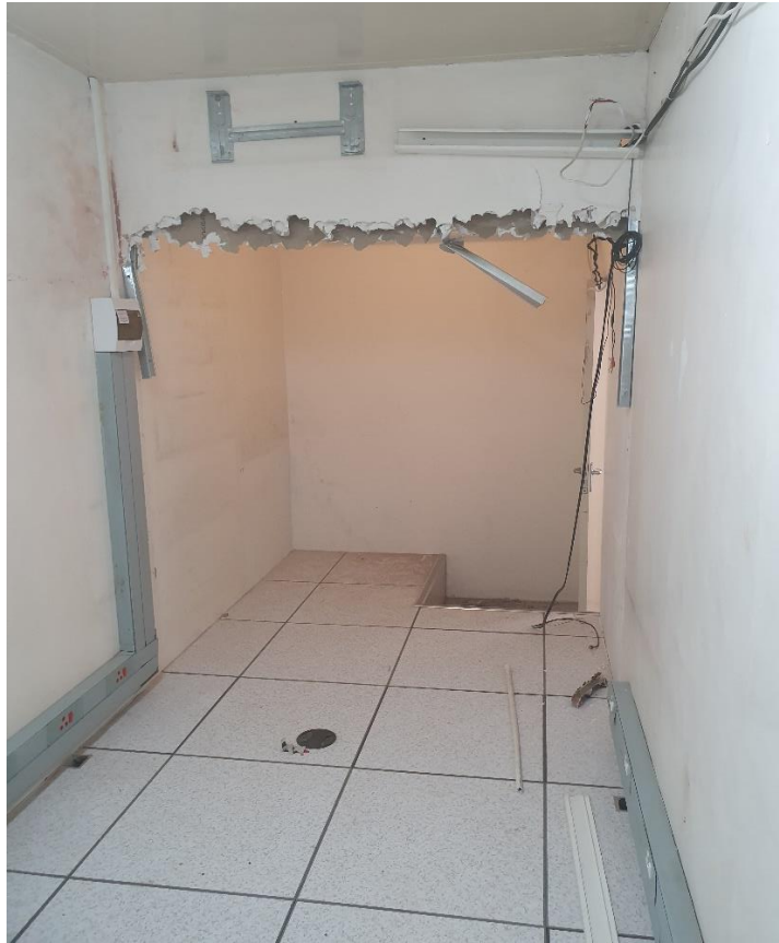
Figure 4-32: Dry wall in server room
