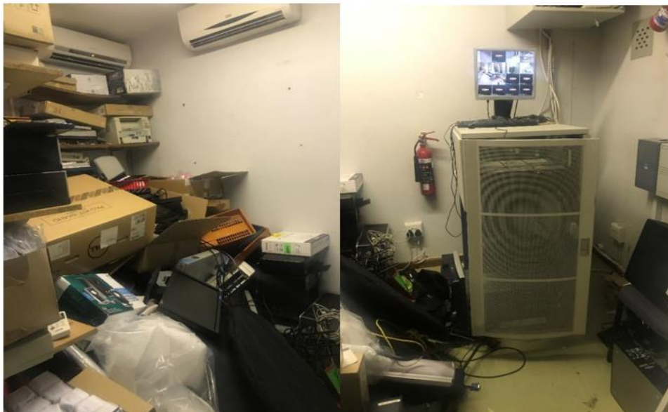
Figure 4-36: Old server room Photographer: Researcher (2020)
