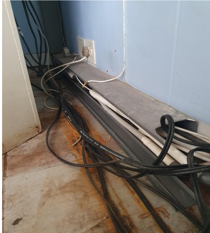
Figure 4-35: Networking and cooling assets (Photographer: Researcher 2020)
