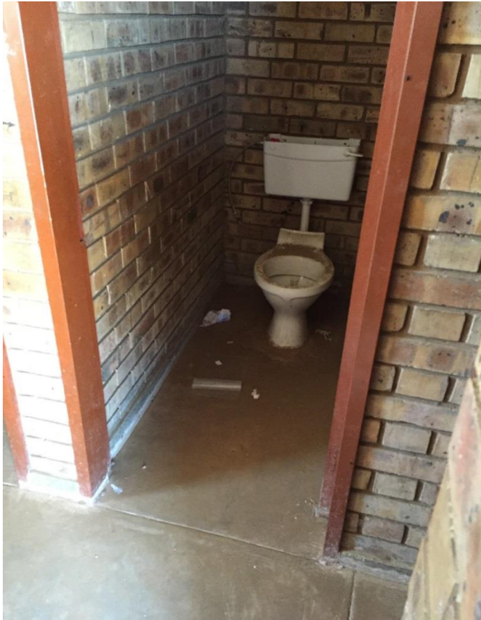
Figure 6: Burgavilla Primary's toilets (not wheelchair accessible)
