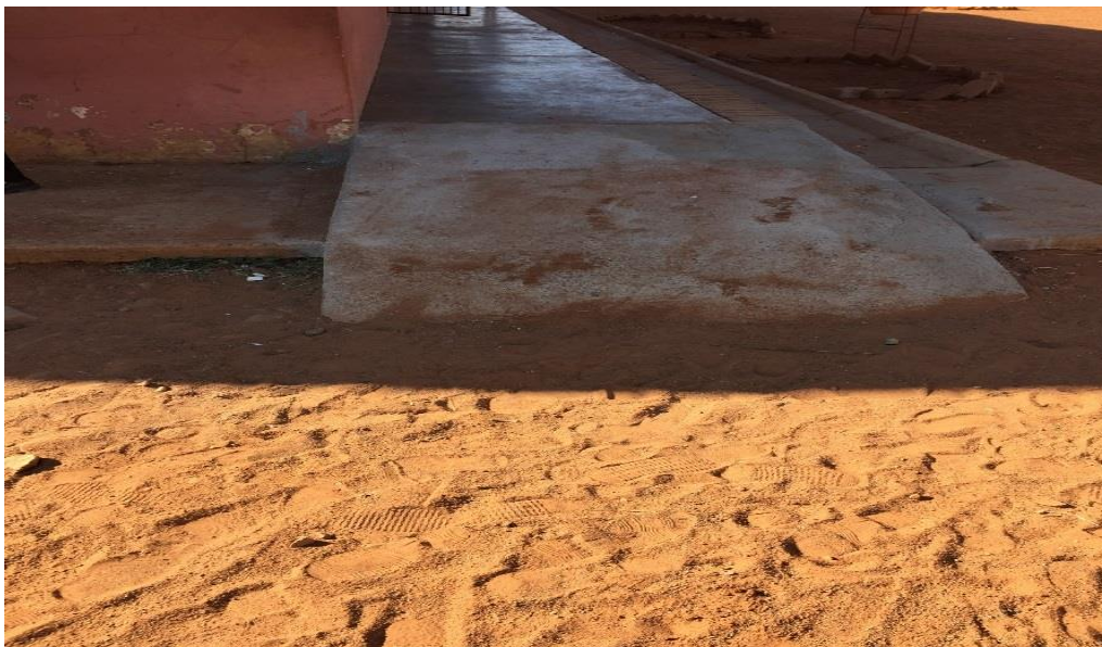
Figure 4: Makoti Primary's ramps (without safety rails)
