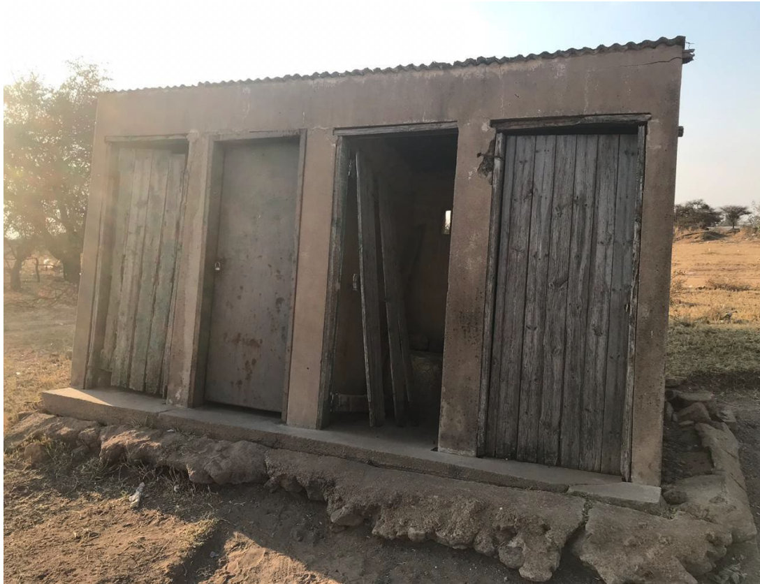
Picture 4: Toilet and doors collapsing
