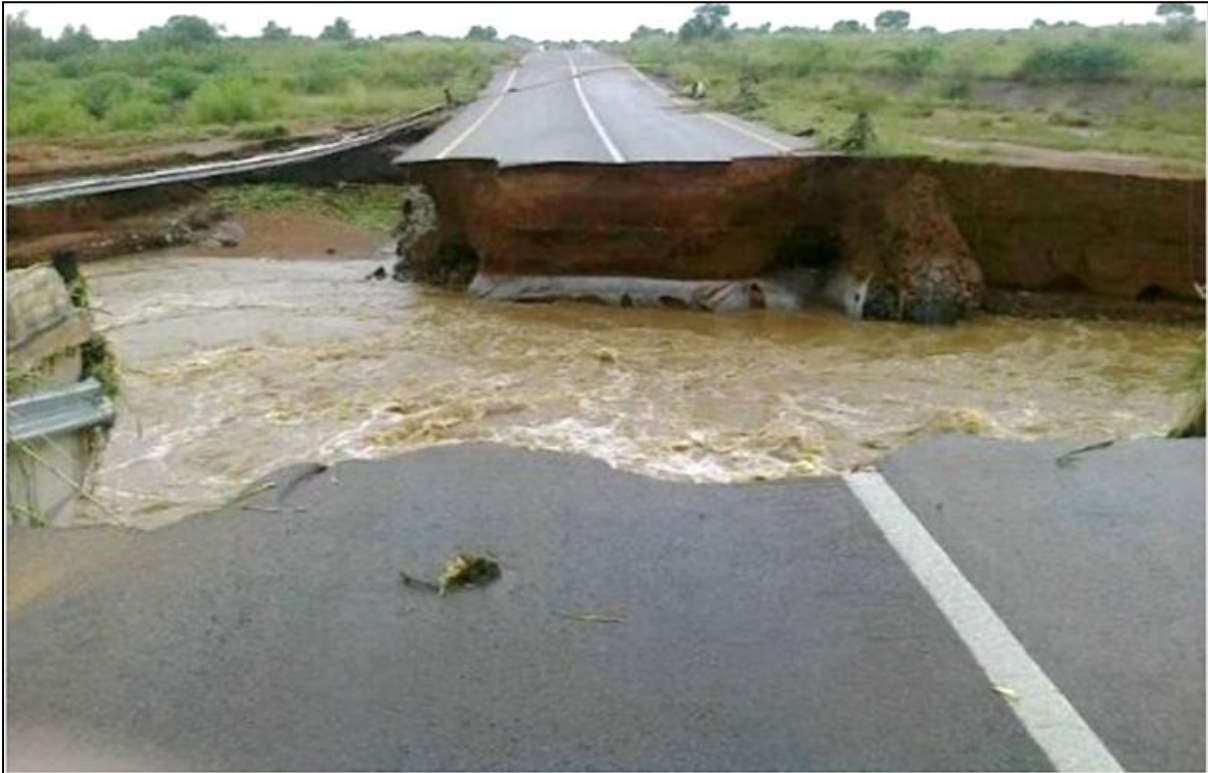
Figure 2.2: The collapsed Mabopane road and bridge
