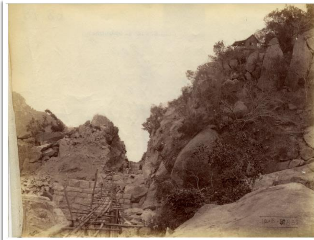
Figure 32 View of the construction of the bridge at KM 85, with a supervisor's hut top right, 1891. Photo: Het Zuid-Afrikahuis Map68-18 1178.
