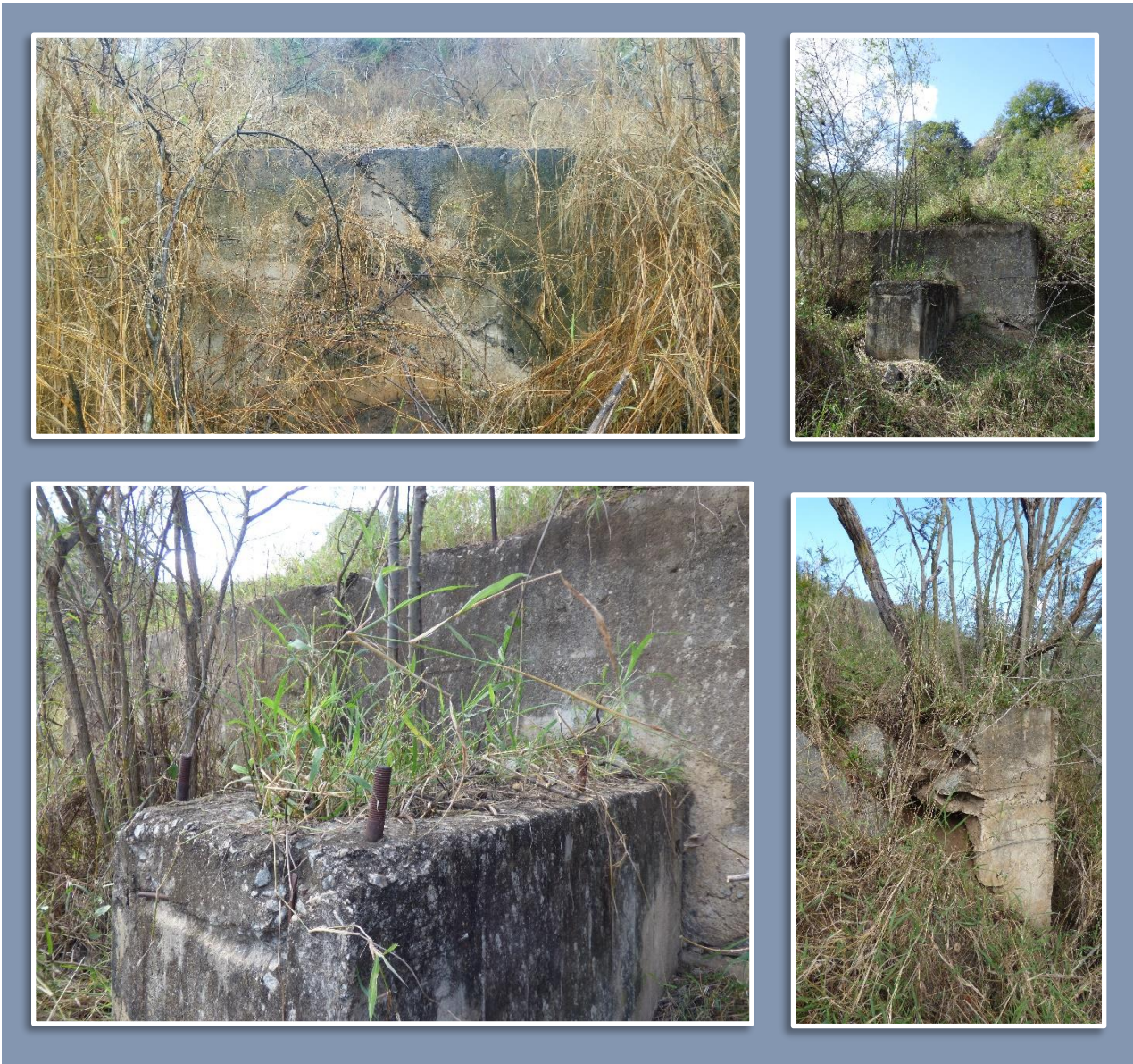
Figure 69 Detail of the loading platform with machine mount screws at KM 93 Bridge. Photos: H. Fivaz.
