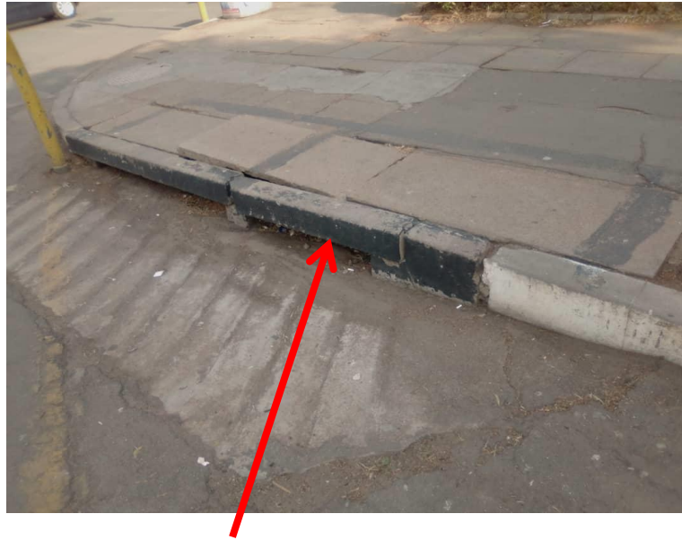
Figure 4.11: A catchpit entrance without a screen cover in the Bulawayo CBD
