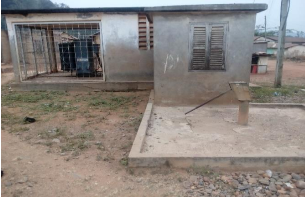
Figure 6.5: Non-Functional Borehole, Abompekrom
