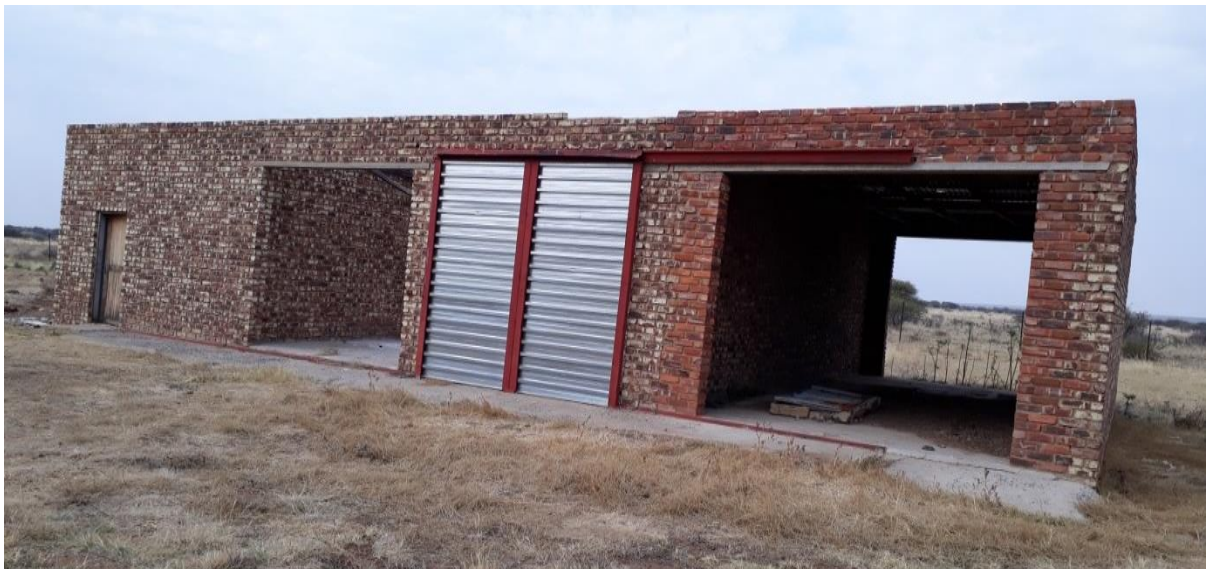
Figure 5.14: Incompletely built farm storage room
