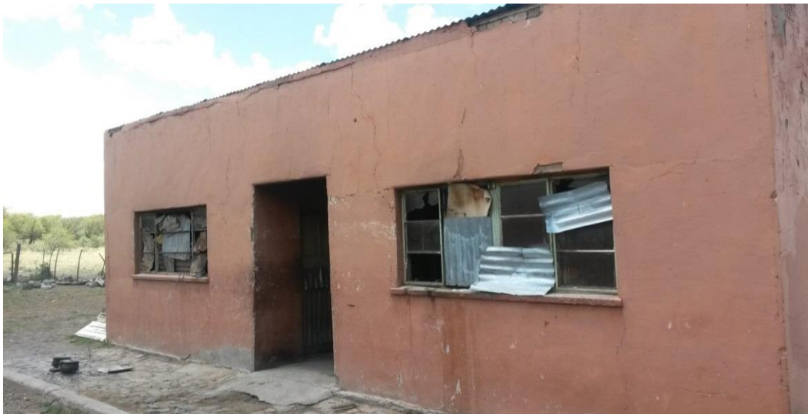
Figure 5.9: Dilapidated farm dwelling on the CPA's land
