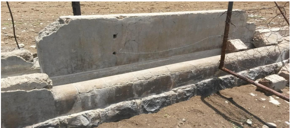
Figure 5.11: Derelict water trough on the CPA's land
