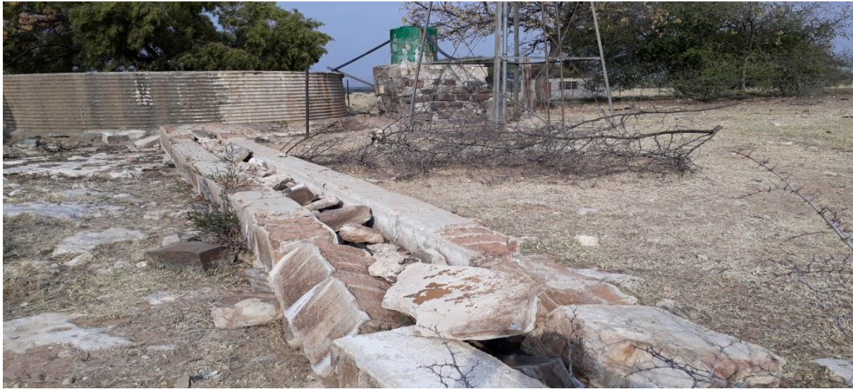
Figure 5.17: Water infrastructure: Reservoir and windmill
