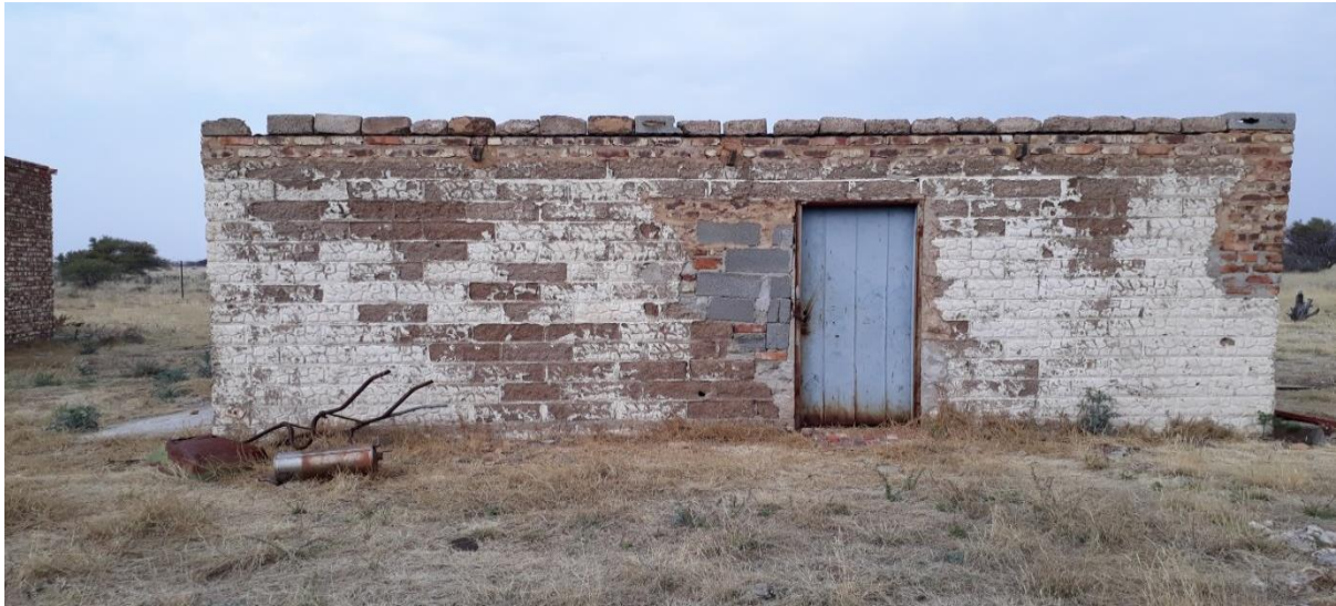
Figure 5.13: Dilapidated farm storage room
