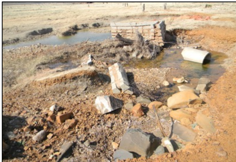
Figure 48: Water Infrastructure in need of maintenance
