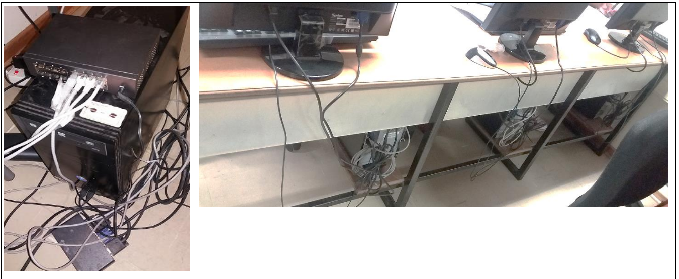
Fig 4.4: Network challenges in some computer laboratories
