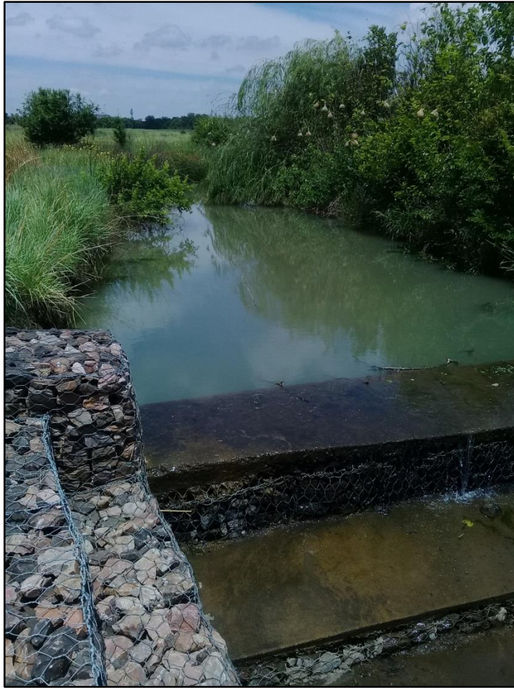
Figure 7.1: Gabion built at Colbyn Valley Wetland supported by Working for Wetlands Programme, a programme of the Department of Environmental Affairs (Source: Author, 2017).
