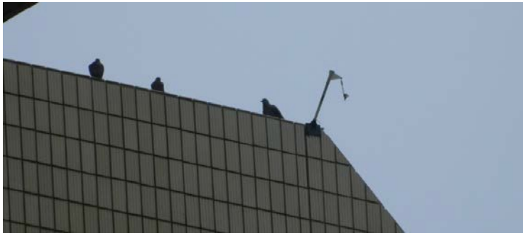
Figure 40: An ineffective broken Fire Flag on OR Tambo building at University of South Africa's Muckleneuk campus
