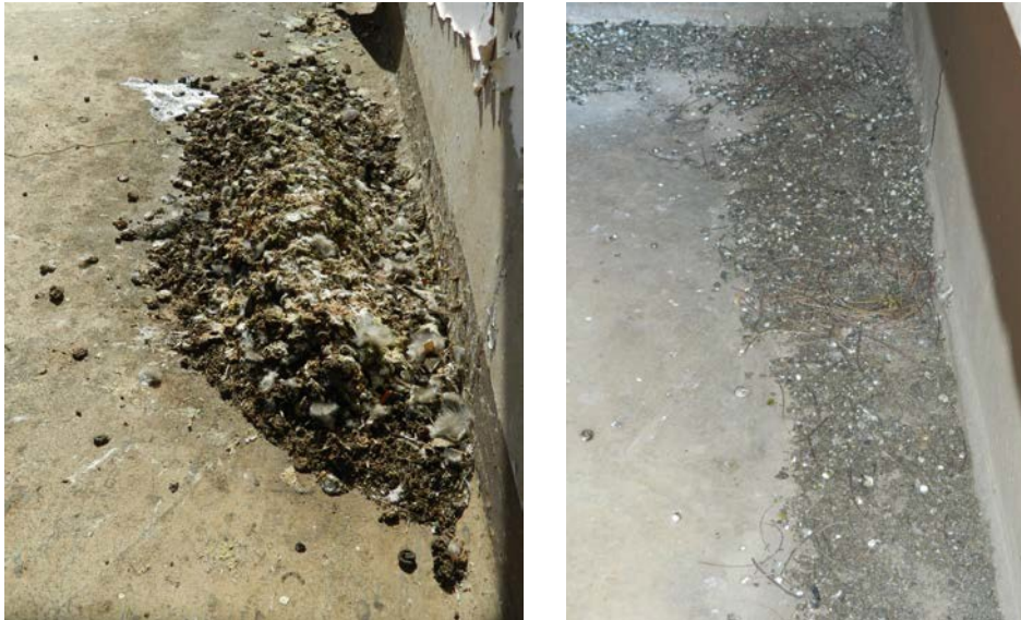
Figure 32: Pigeon dropping and debris accumulation on balconies of OR Tambo building on the University of South Africa's Muckleneuk campus
