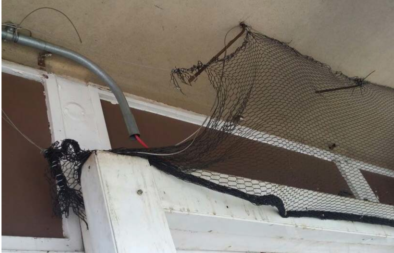
Figure 36: Redundant netting aimed at excluding pigeons from sections of the Theo van Wijk building on the University of South Africa's Muckleneuk campus
