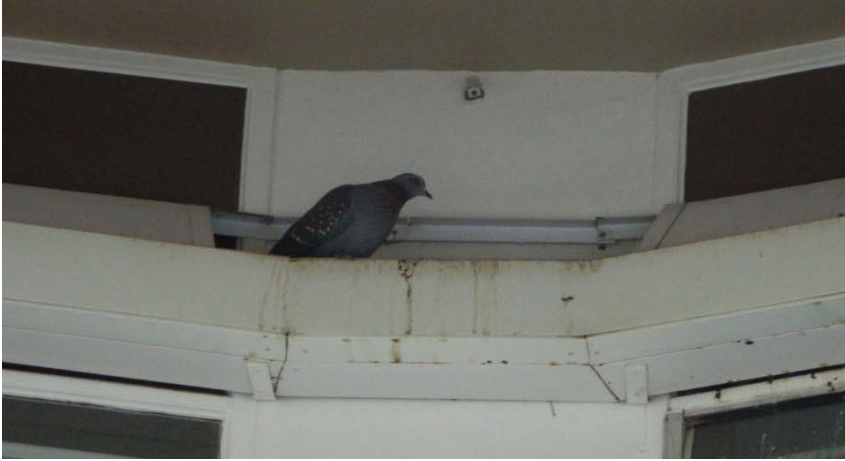
Figure 44: Speckled Pigeon nesting in an open cabling duct (trunking) of AJH van der Walt building at the University of South Africa' Muckleneuk campus
