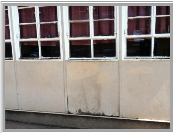
Figure 4.3: Water damage on classroom and broken windows
