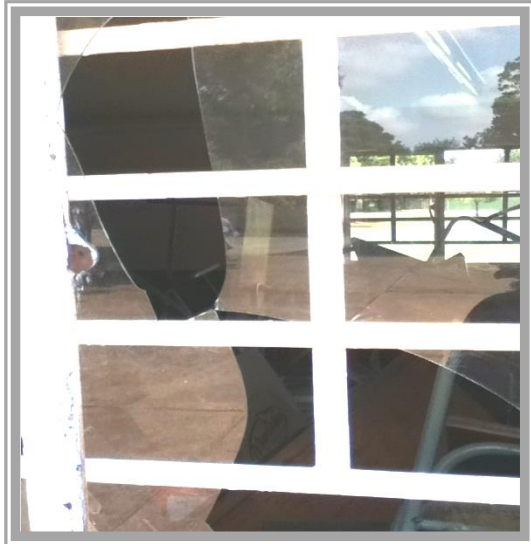
Figure 4.20: Broken window in a classroom due to poor maintenance
