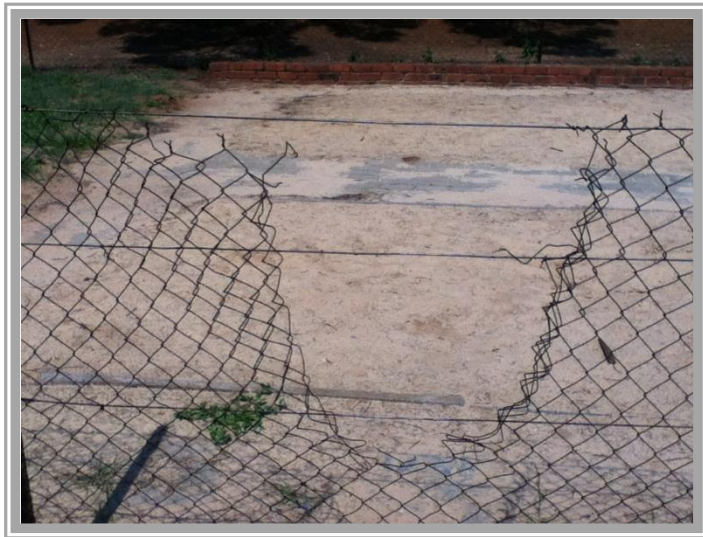
Figure 4.17: A broken fence presenting a physical hazard on a playground
