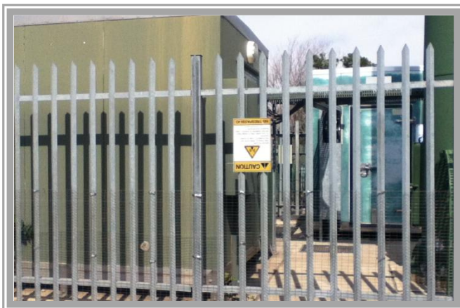
Figure 5.3 : Electrical hazards need to be effectively fenced off and marked
