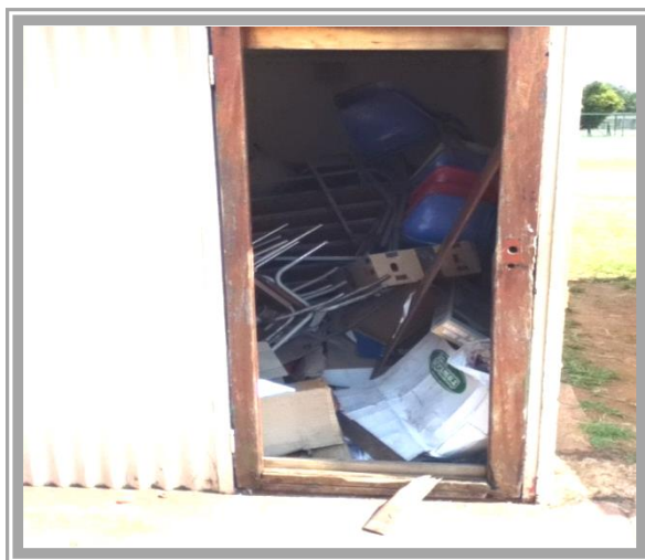
Figure 4.27: Maintenance/storage facility on school grounds without a door
