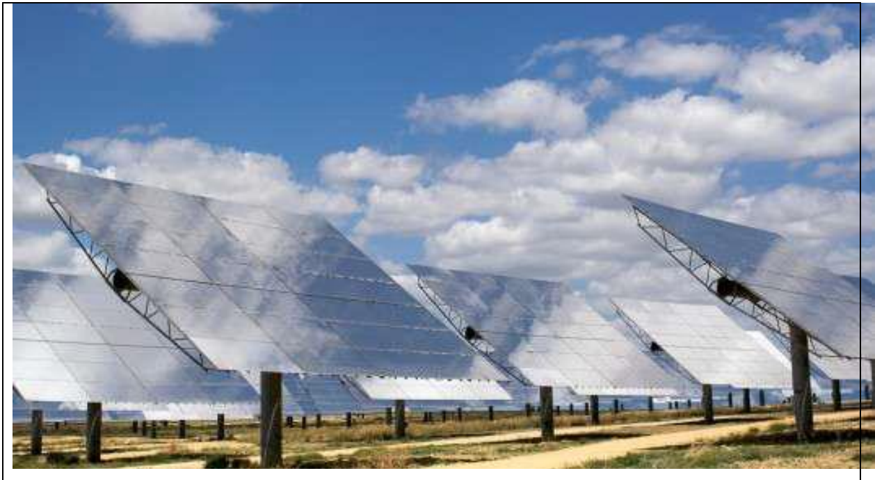
Figure 4.3: Ekurhuleni Solar photovoltaic (PV) plant
