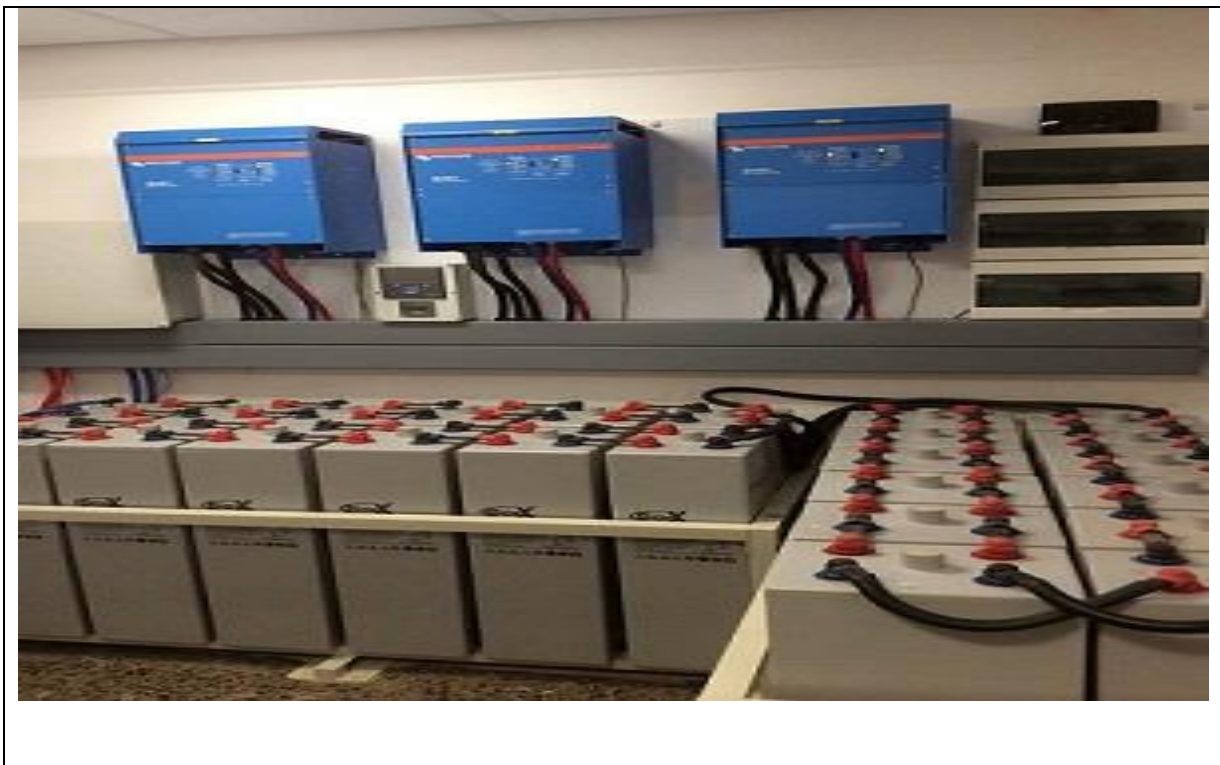
Figure 4.7: Batteries for the storage of excess generated solar electricity
