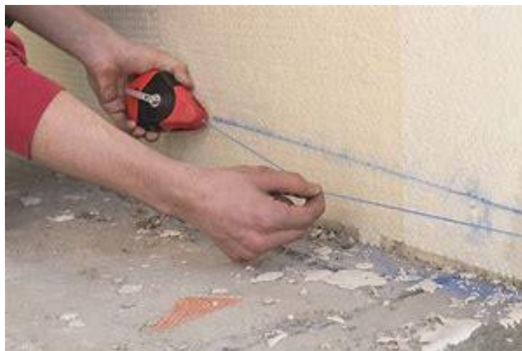
Figure 2-19: Method of the chalk line to draw a straight line in construction (Stock photo, open source).
