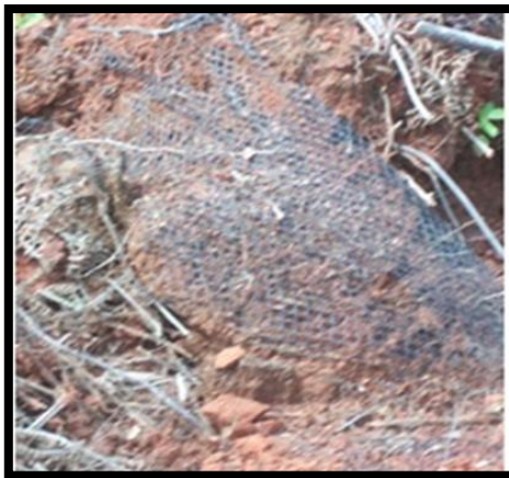
Figure 4.5 Damaged wire mesh of an ineffective gabion wall along the R523 road due to landslide re-occurrence
