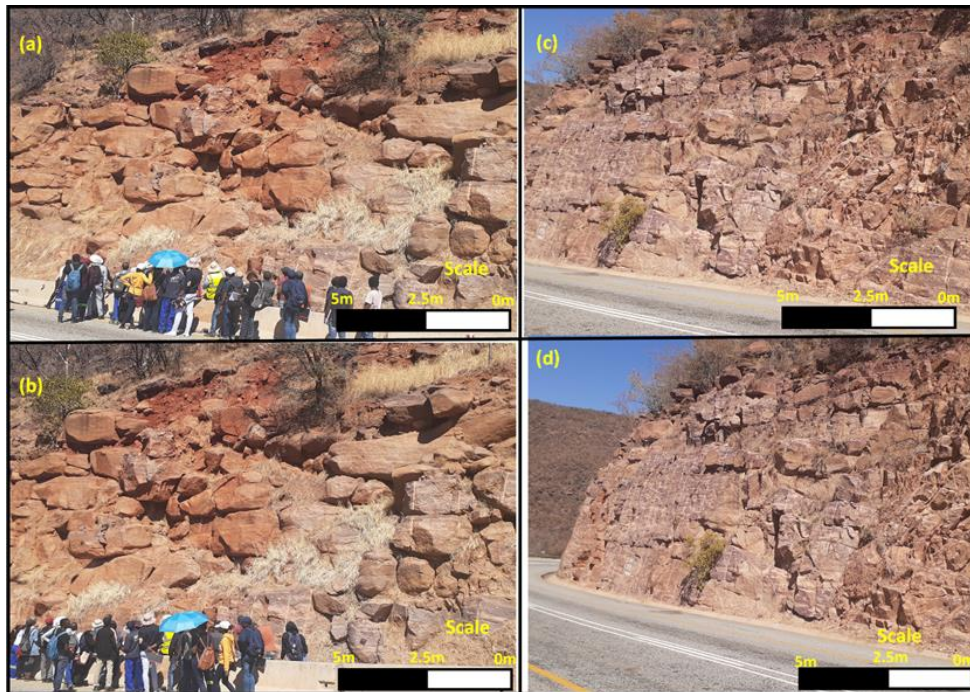
Figure 7.2 Poor quality rock mass in site 1 with loose rock at the upper part of the road slope and very steep slope
