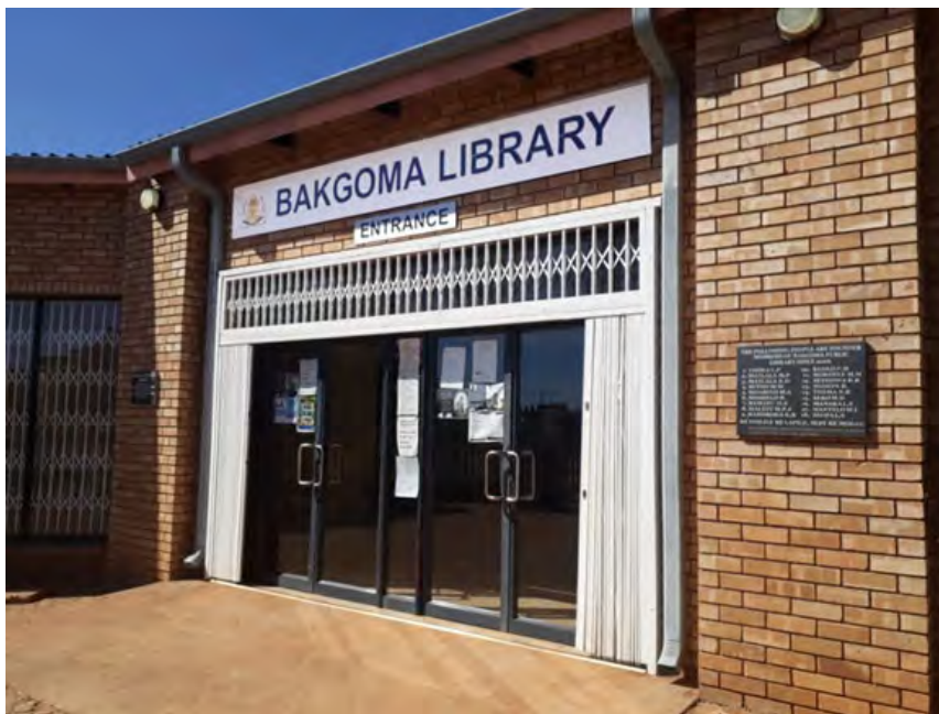
Fig.2-3. View of the new Bakgoma Library showing memorial plaque Source: Lekanka Petrus Thoka
