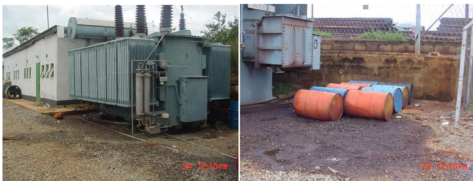
b) Leaking transformer oil drums c) Used transformer storage site
