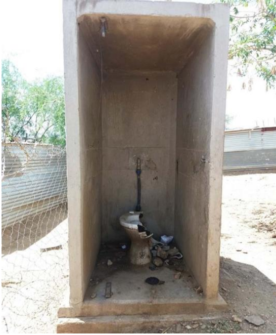
Figure 4.6: Vandalism of communal toilets (The Namibian Sun, 2020)
