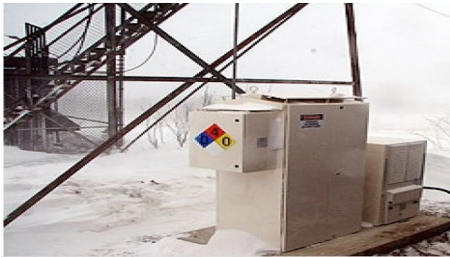
Figure 2.16. Backup power source (Olabi et al. , 2022).
