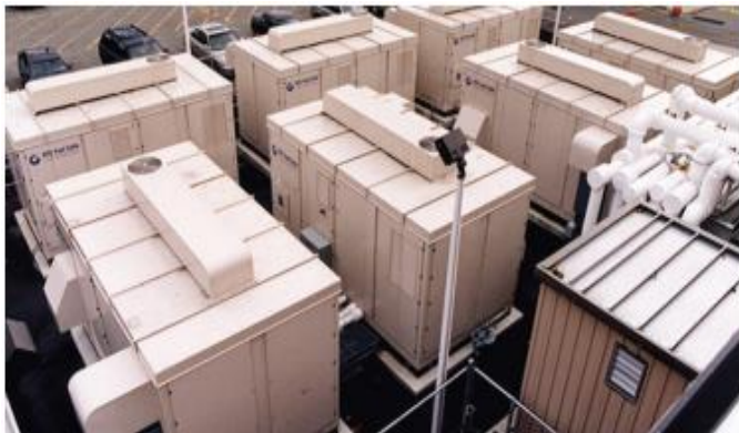
Figure 2.14. CHP building (U.S. Department of Energy, 2016a).
