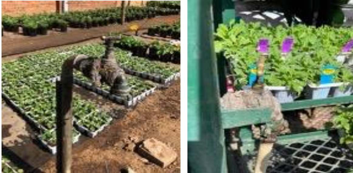
Photo 27 – 28 – Material is used to prevent taps from freezing
