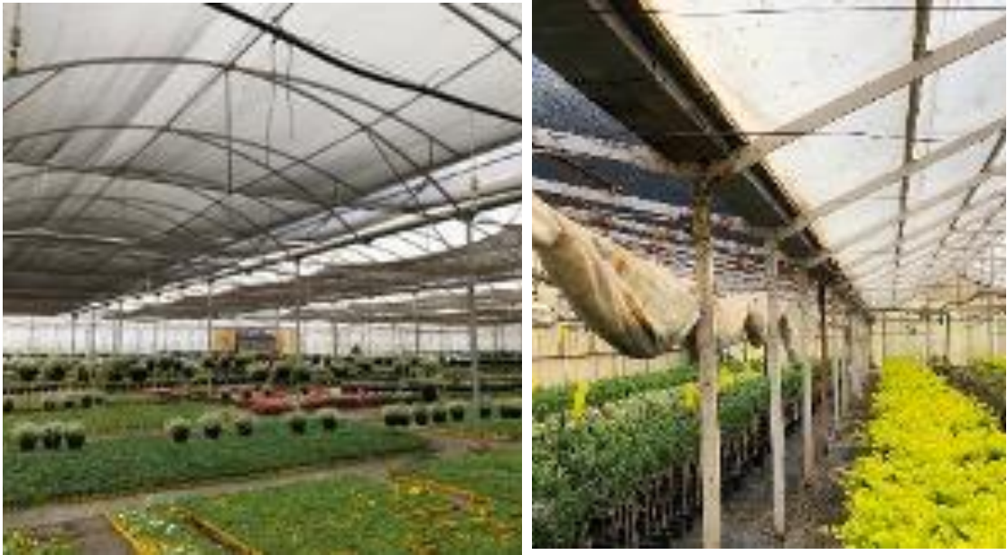
Photo 15 – 16 – Greenhouse insulation and screens for temperature control
