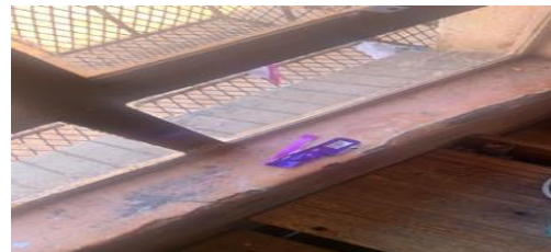
Picture Z: Solid waste on window Security bar
