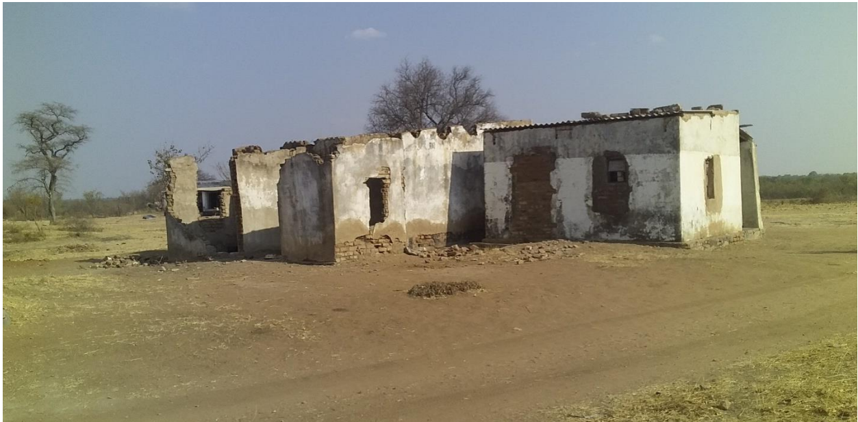
Figure 5.2: A dilapidated general dealer shop, butchery and bar building where students used as classrooms.
