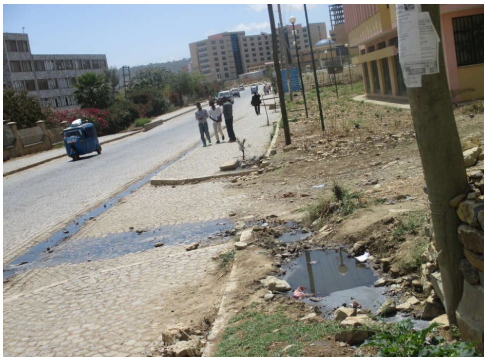
Figure 6: Liquid waste exploding from the septic tank in condominium houses, near Regional Administration Office, Mekelle city
