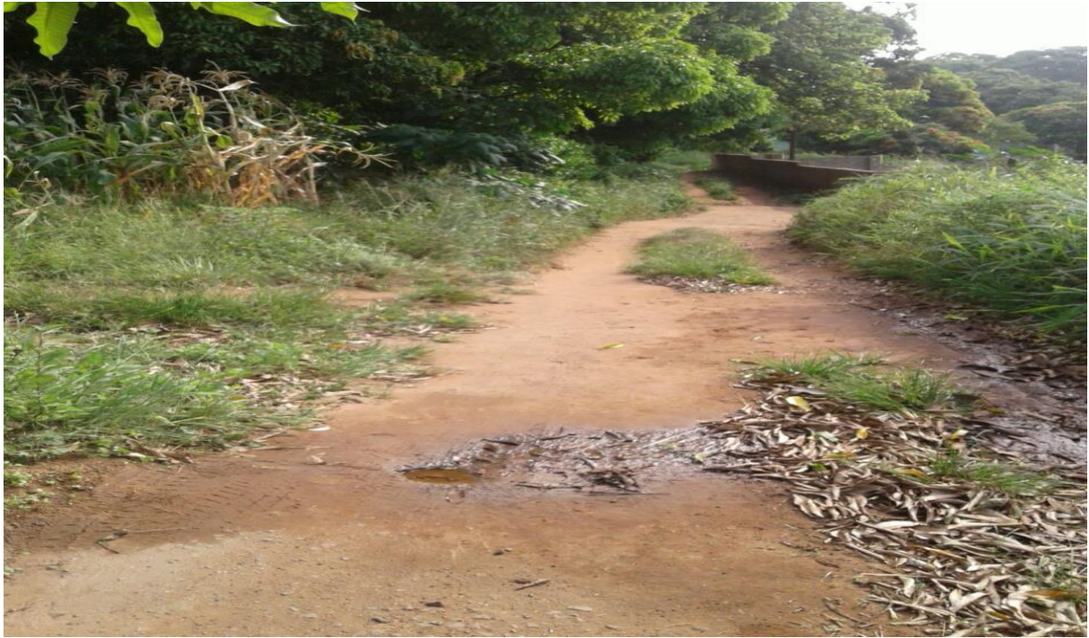
Figure 7.3: Burst municipal water pipe that has not been reported or fixed, making traversing of this road slippery and dangerous, while also contributing to soil erosion. ( Source: Own).
