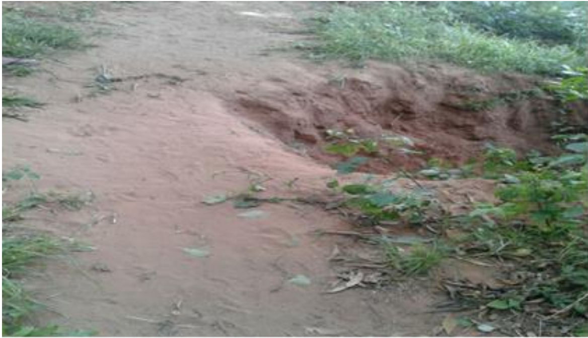
Figure 7.1: Route with visible soil erosion, used as a shortcut by school commuters attending Umnganiwakhe High and Umcothoyi High. (Source: Own).
