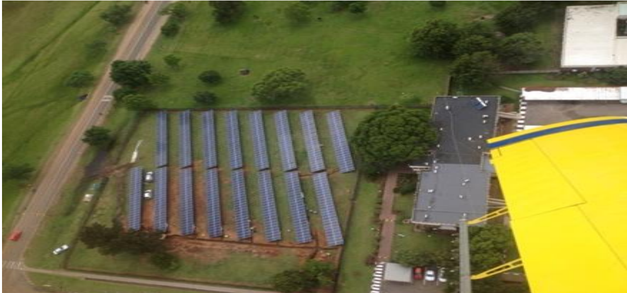
Figure 4.12: Solar photovoltaic at Kriel Colliery
