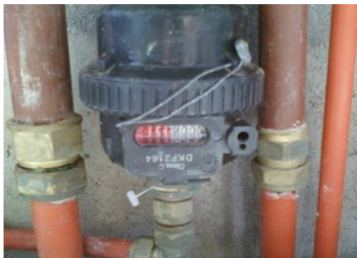
Figure 8: One of the 15 mm Kent mechanical flow meters inserted on the TEARS potable top-up system.
