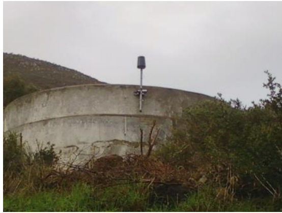
Figure 9: The electronic bucket-type rain gauge installed at the TEARS study site.
