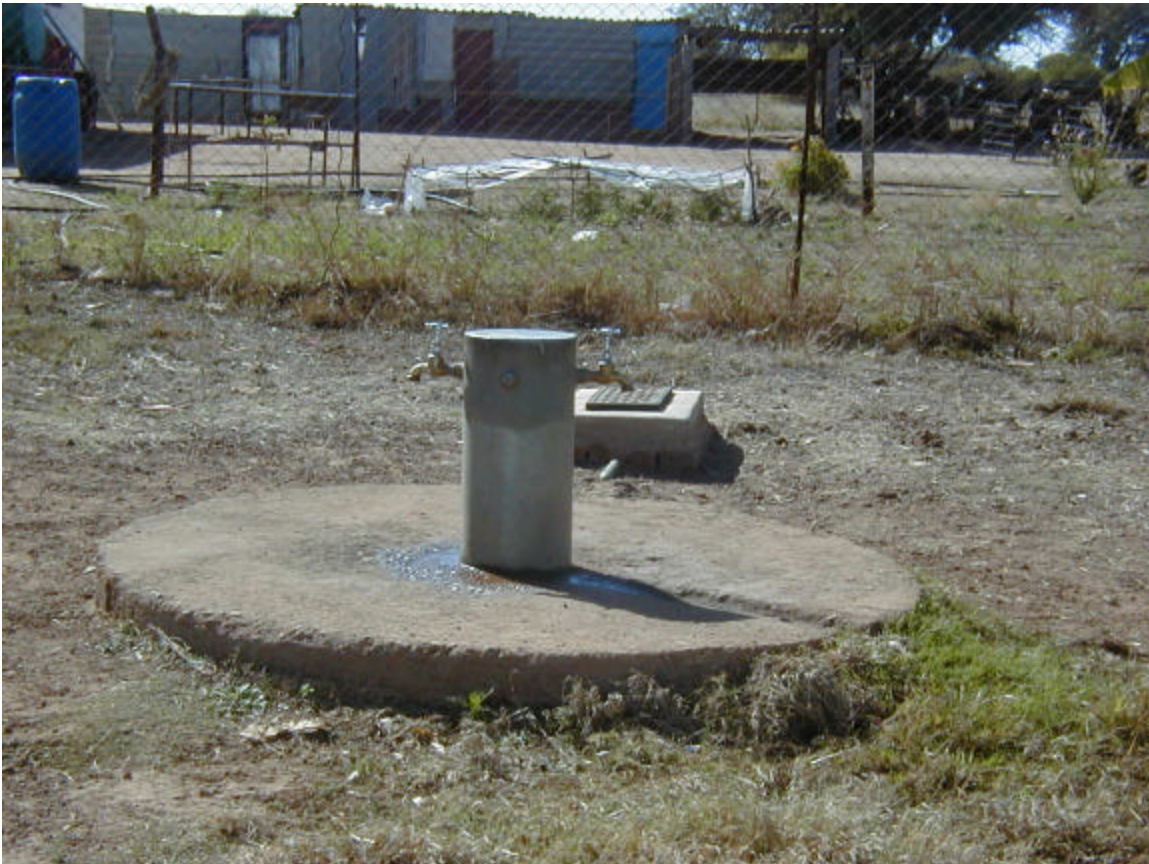
Figure.5 Street taps in Moruleng
