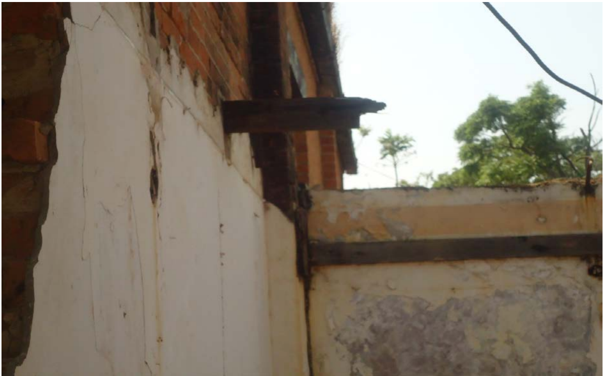
Plate 6: The dilapidated part of the building, seen from one of the rooms (part 10 on the sketch-map).
