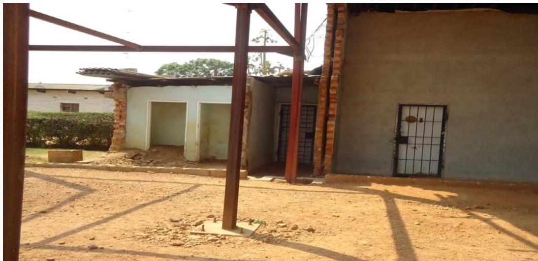
Plate 2: Showing part of the demolished old structure and the initial reconstruction works (in portal frames) by the SDA Church.
