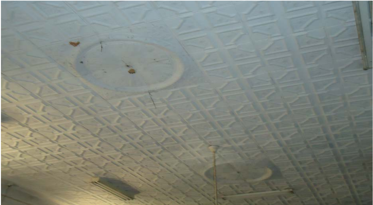
Plate 7: The remaining part of Ceiling Board.
